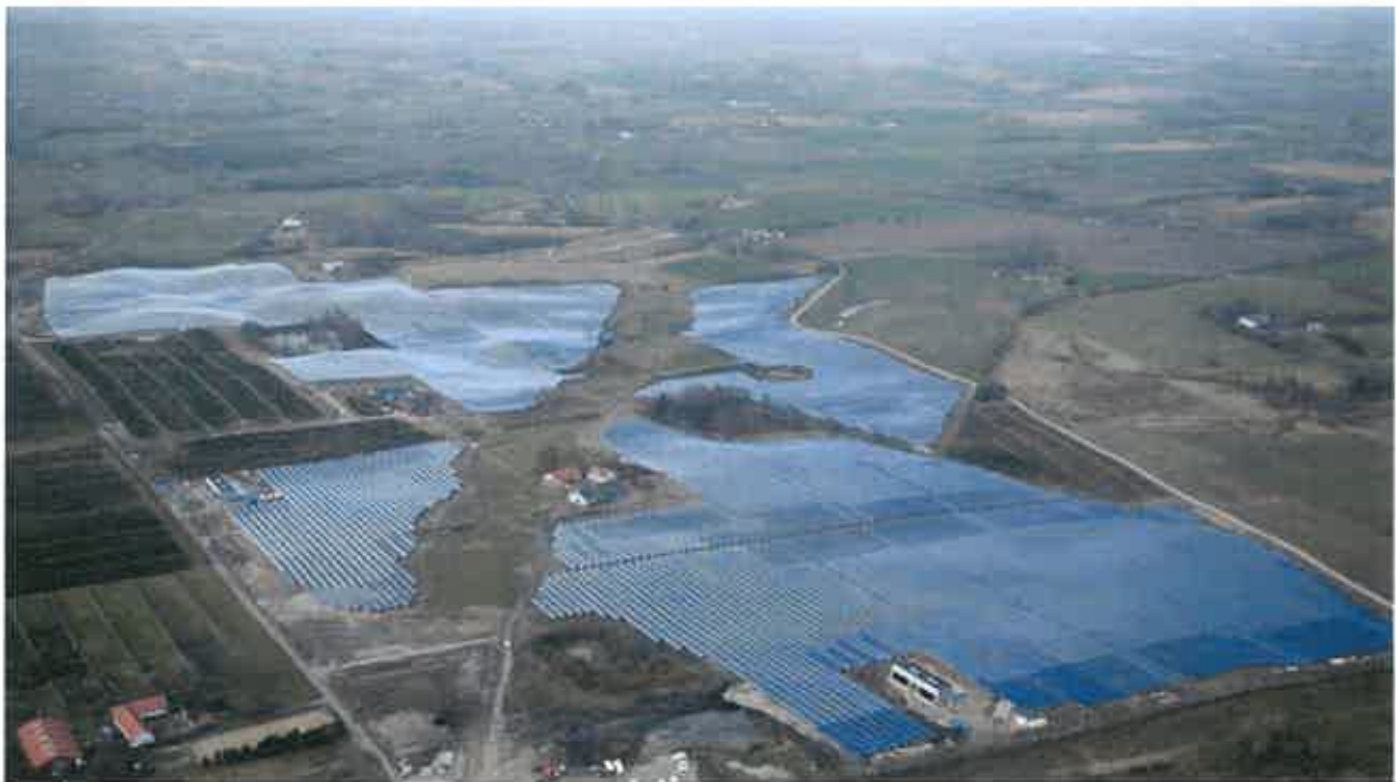
Figure 3: Solar thermal district heating plant in Silkeborg, Denmark [4].
